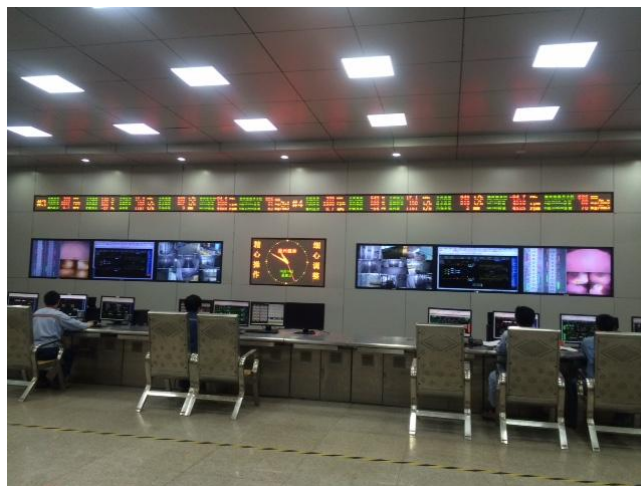
Figure 3: Control room of 3# and 4# power plants
